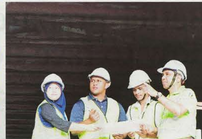
Yusni Shahadan (right) explaining to the young engineers on the work progress at the Merdeka Station KVMRT underground site.
