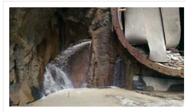
Water inrush through the end wall of the Pasar Rakyat station box from a network of karst features
